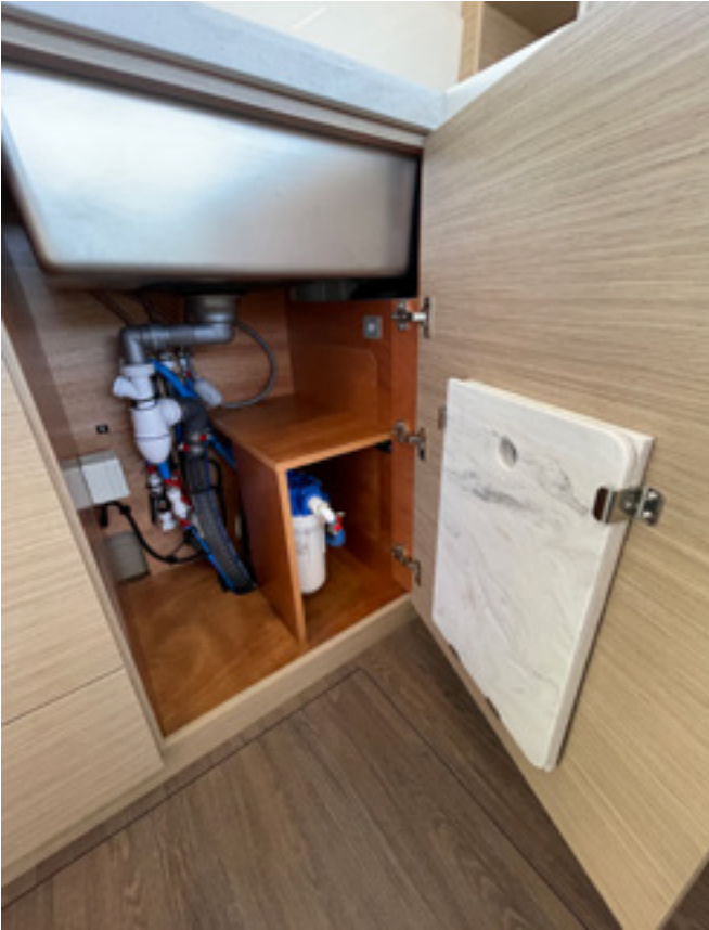
Non contractual picture Located under the galley sink
